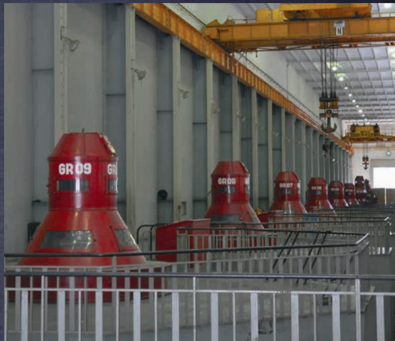
Machine hall of HPP Edéa
