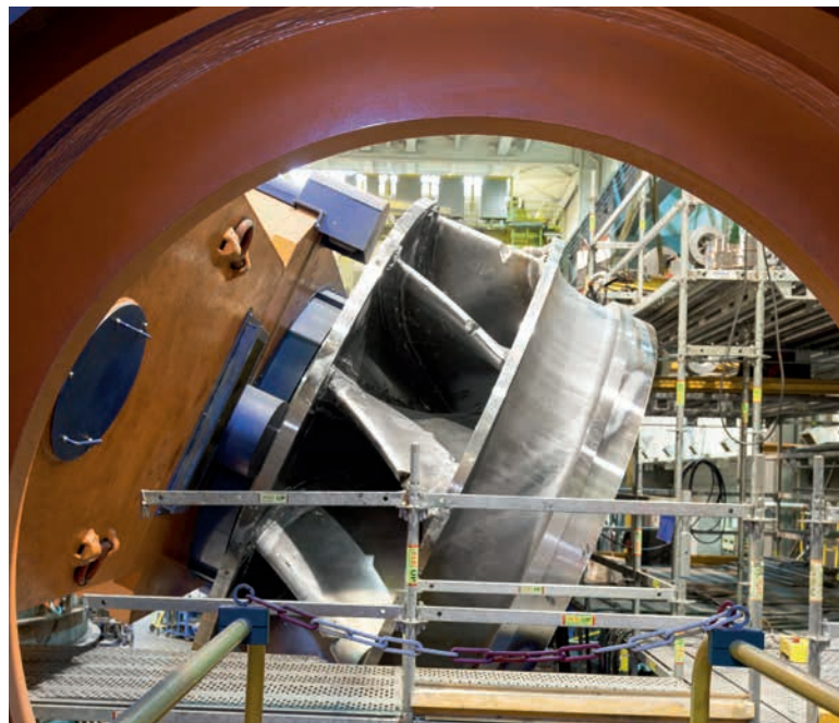
Francis turbine for HPP Laúca
