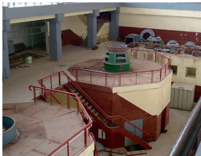
Machine hall of HPP Djoué
