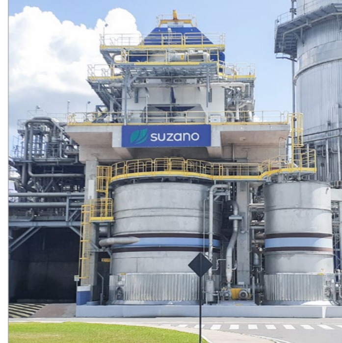
A DD-Washer was installed in the brownstock washing between existing wash presses.
